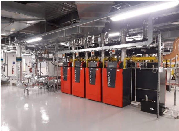
Figure 5 - Replacement Boilers at QMH, Dunfermline
