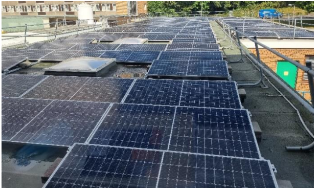
Figure 6 - Photovoltaics at VHK, Kirkcaldy
